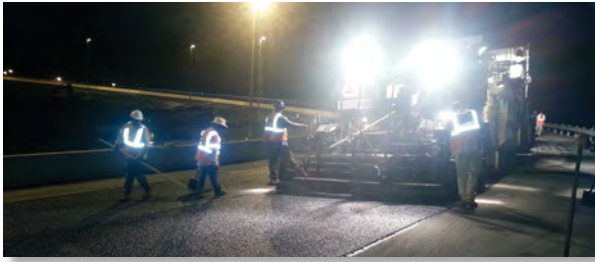
PGA ramp resurfacing at night for minimal traffic impact and improved safety.
