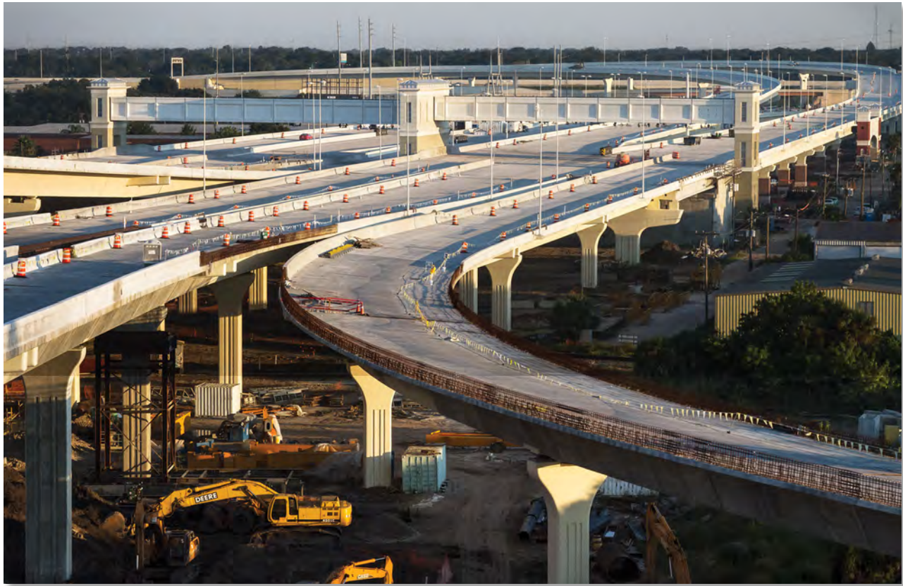
The I-4 Connector is an integral part of the Tampa area transportation infrastructure. The facility is equipped for AET and hosts the longest spanning toll gantry in the state. The facility opens to traffic in January 2014.
