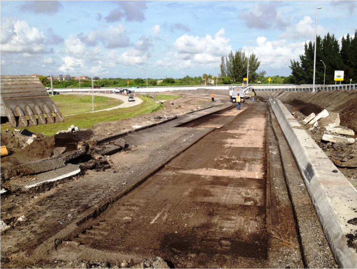
Figure 10 – Utilization of Excessive Asphalt Thickness at Bridge Approaches
