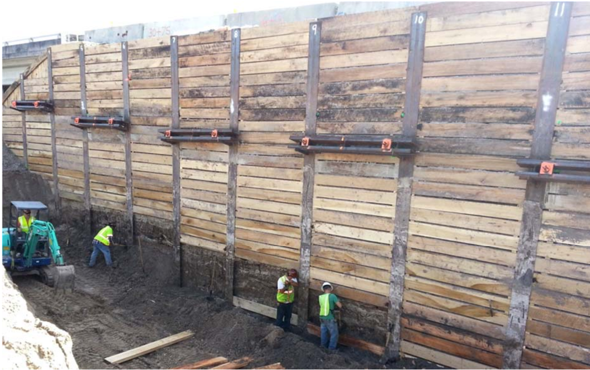
Figure 3 – TW-1 Lag Wall with Soldier Pile Construction in Lieu of Permanent Sheet Pile
