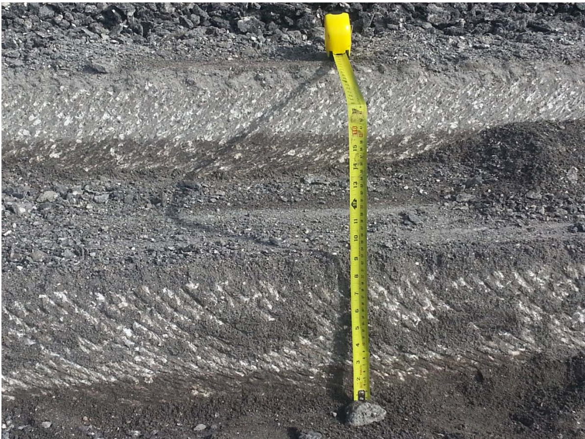
Figure 9 – Excessive Asphalt Thickness at Bridge Approaches
