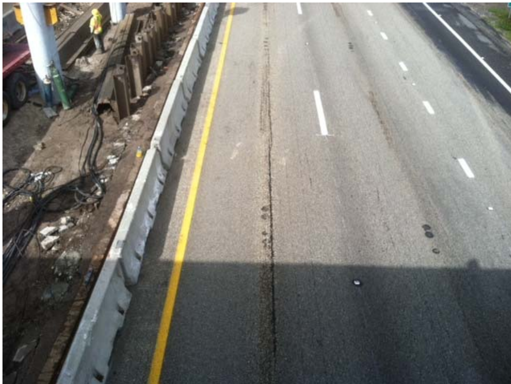
Figure 8 – Northbound Mainline cracking Lane R-1 (shifted) adjacent to Median Pier 2
