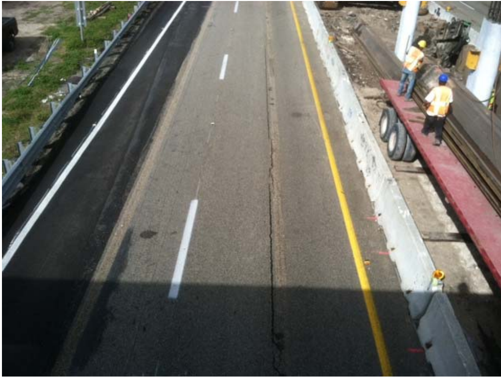
Figure 7– Southbound Mainline cracking Lane L-1 (shifted) adjacent to Median Pier 2
