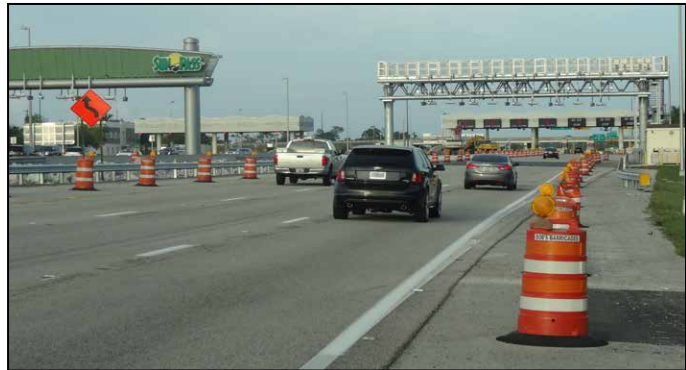
The Sawgrass Expressway is the second facility after SR 821 (HEFT) to be converted to AET.
