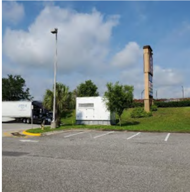
Site 9 – Duke Energy/Target East of diesel generator looking west towards SR 429
