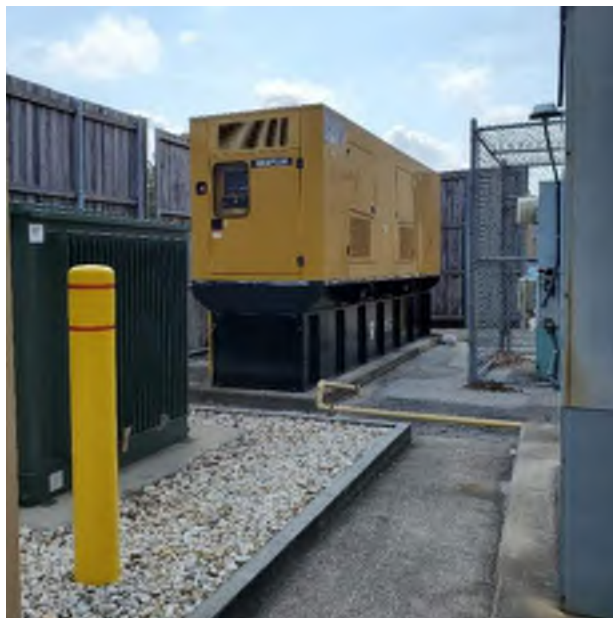
Site 10 – Publix Diesel Generator with base tank located at northwest corner of Publix
