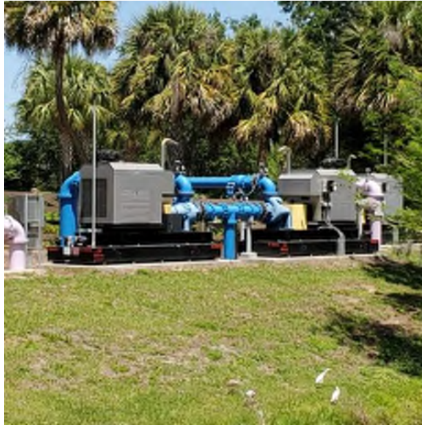
Site 17 – Three diesel generators with base tanks South of Western Way looking northeast
