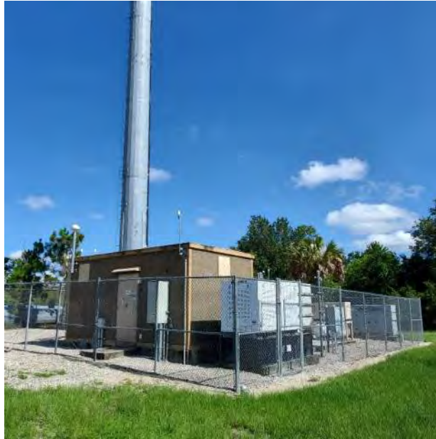
Site 14 – SBA Cell Tower Southeast corner looking northwest
