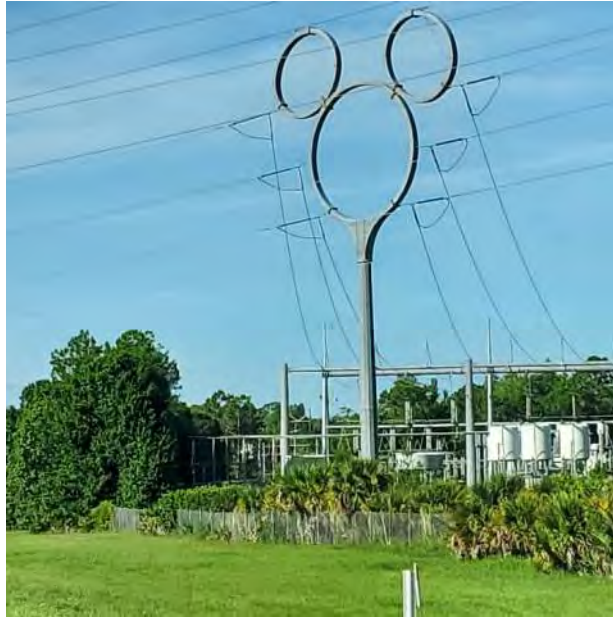
Site 20 – Osceola Substation Southeast of substation looking northwest
