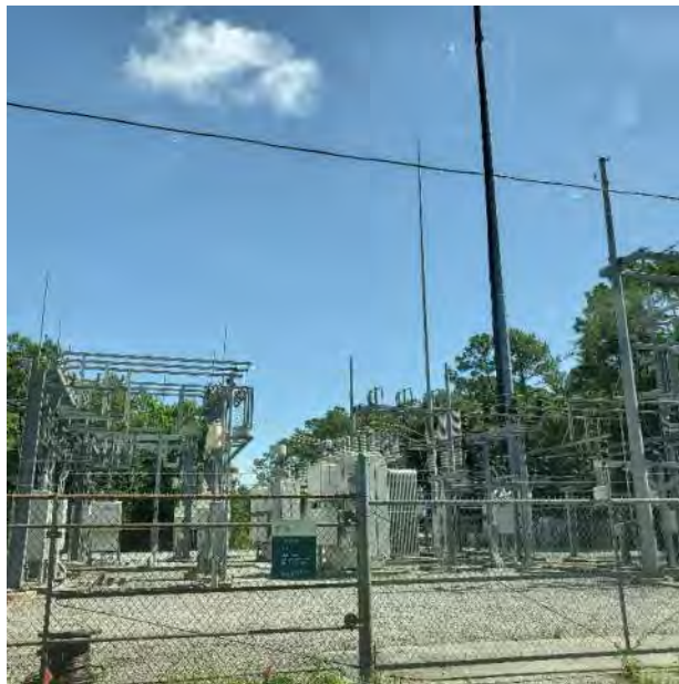
Site 21 – Lake Wilson Substation South of substation looking north
