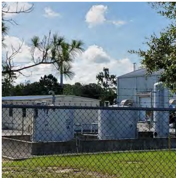
Site 11 – FGT Davenport Compressor Station Tank farm in containment
