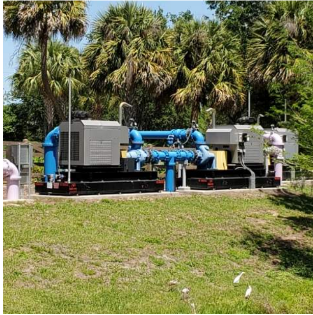
Site 17 – Three diesel generators with base tanks South of Western Way looking northeast
