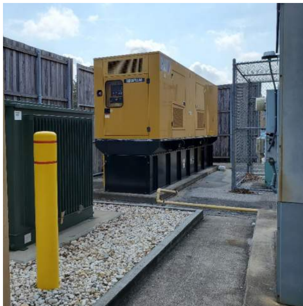
Site 10 – Publix Diesel Generator with base tank located at northwest corner of Publix
