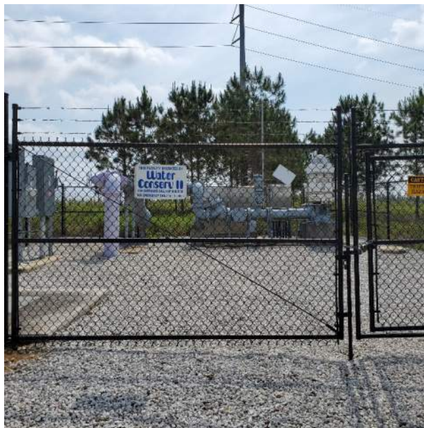
Site 22 – Water Conserve II 3W-01 Supplemental Well West side of facility looking east
