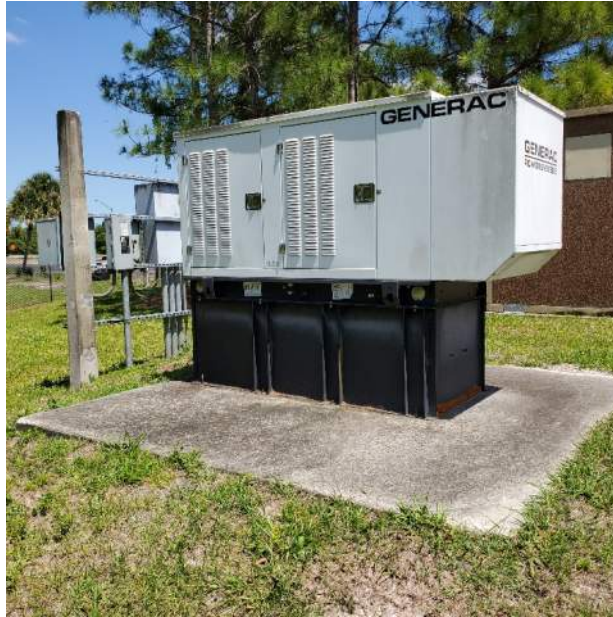
Site 12 – Toll Plaza 5602 Diesel generator with base AST located northwest of Administrative Office
