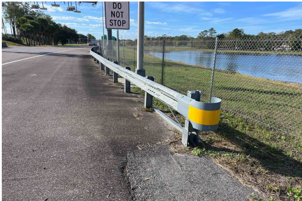
Desired Fence Condition
