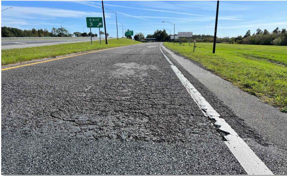
Undesired Pavement Condition - Class III Cracking
