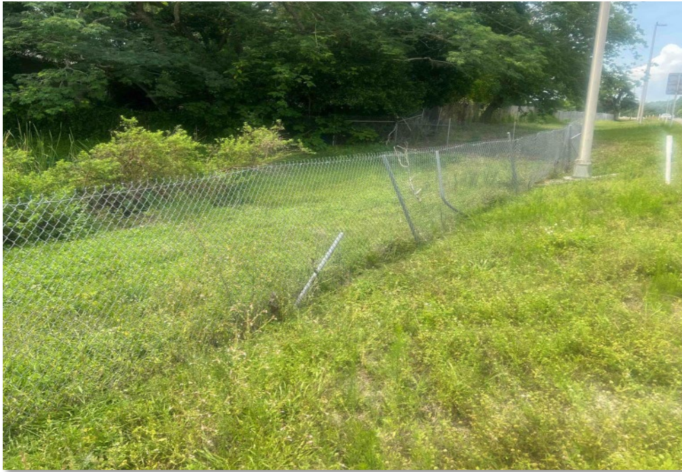
Undesired Fence Condition - Damaged Fence Post
