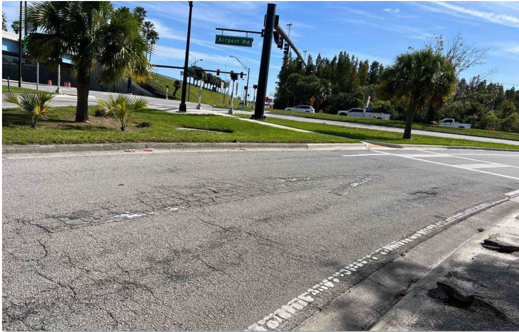
Undesired Pavement Symbol / Cracking
