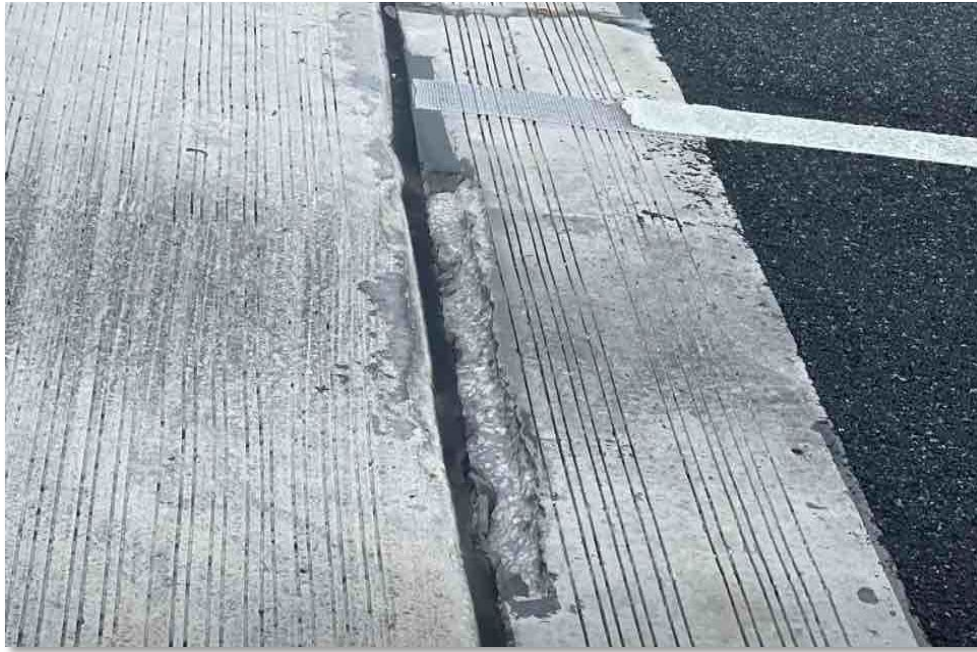
Undesired Joint Condition – Spalled Joint
