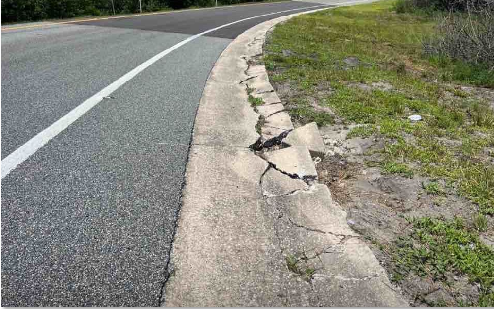
Undesired Shoulder Gutter
